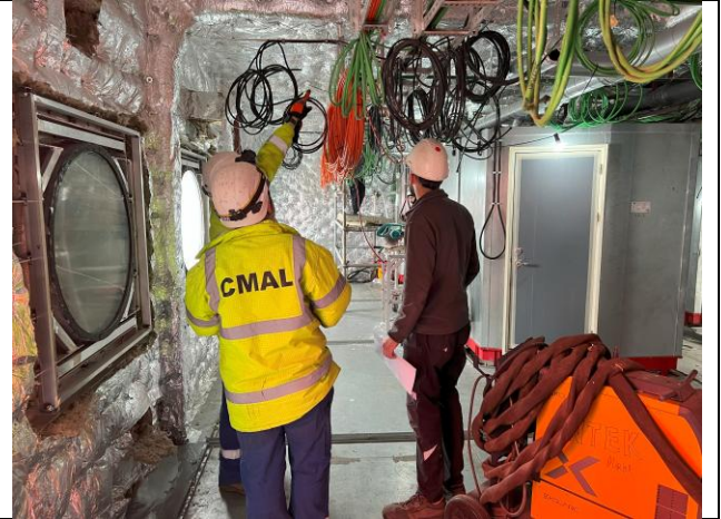
Aft Accommodation Internal
